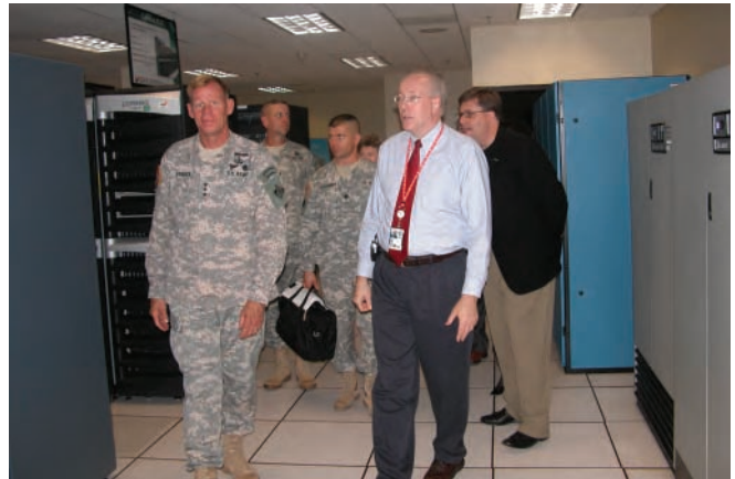
LTG Carl A. Strock (far left) walks through Joint Computing Facility as Dr. Jeffery P. Holland (second from right), ERDC Acting Deputy Director, and John West (far right) discuss supercomputing infrastructure, July 18
