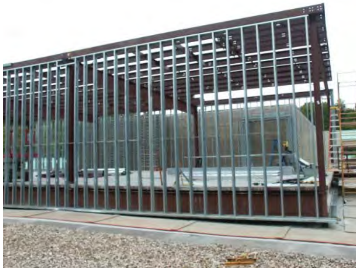
Figure 1. New UPS equipment shelter located on the roof of ERDC Information Technology Laboratory building
